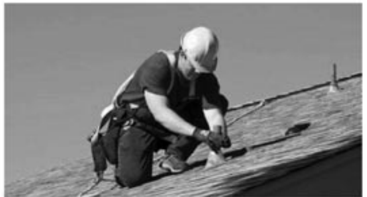
Make Necessary Repairs
