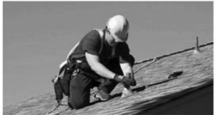
Make Necessary Repairs
