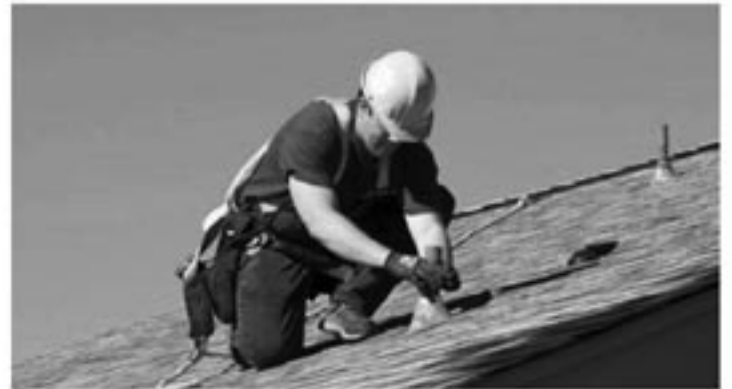
Make Necessary Repairs
