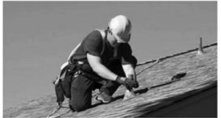
Make Necessary Repairs
