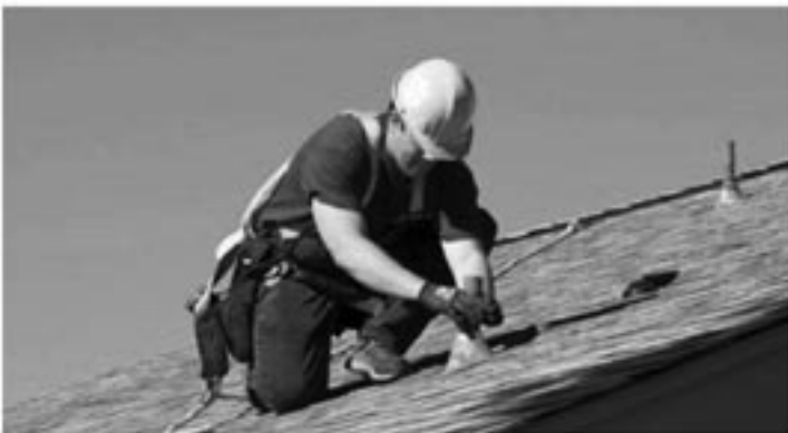
Make Necessary Repairs
