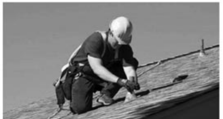
Make Necessary Repairs
