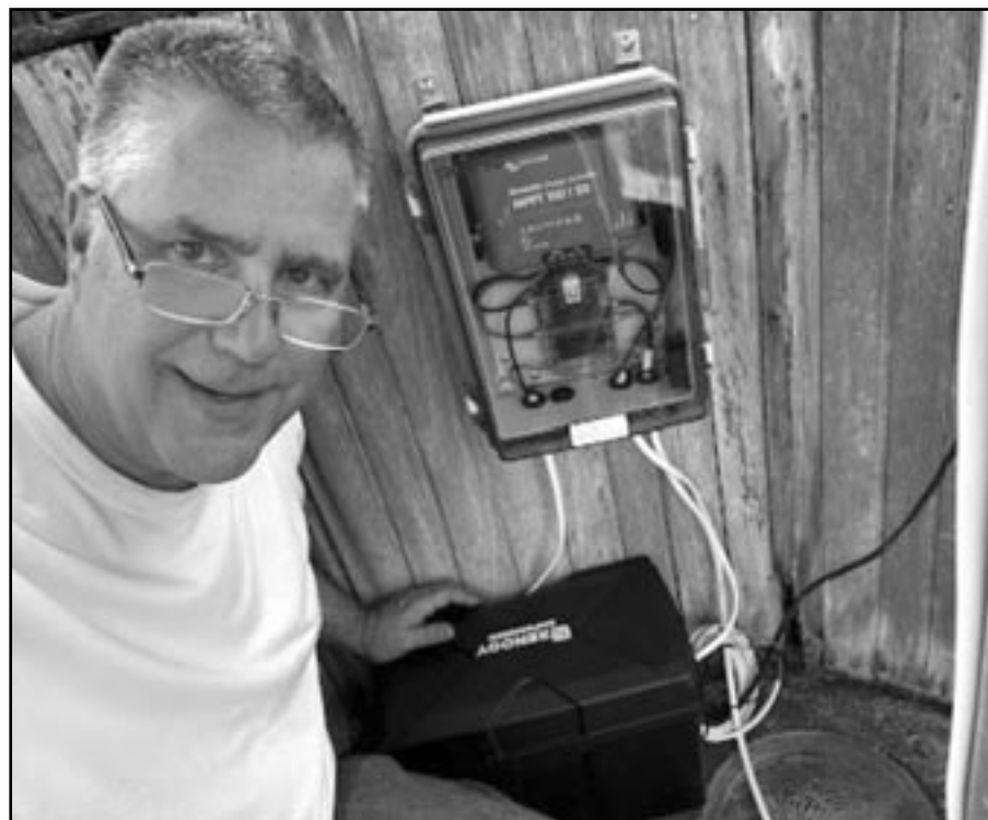
(above) Timothy Canary and his electrical engineering handiwork.
