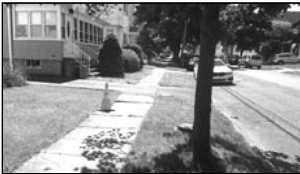
(above) A section of sidewalk along Pershing Ave. that will be repaired and made safer for pedestrians.
