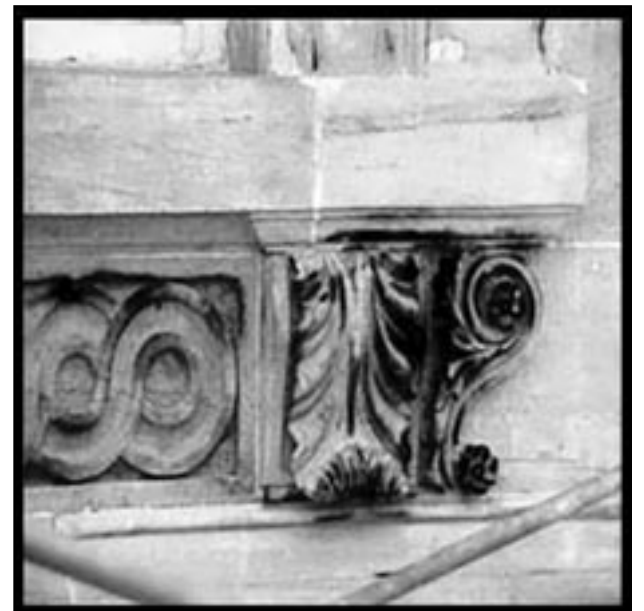
(above) Burn marks on the White House from the War of 1812, uncovered during restorations in 1992.
