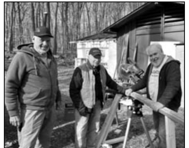
(above) The Pool House under construction; George, Tom and Barry making knee walls for the building.
