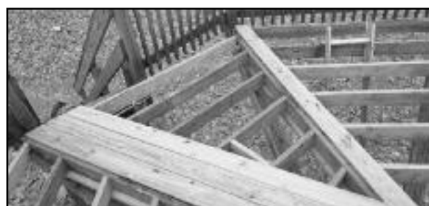
(above) The Dan Beard Tree House at Boy Scout Camp Somers received repairs by the Flintlocks over the winter.
