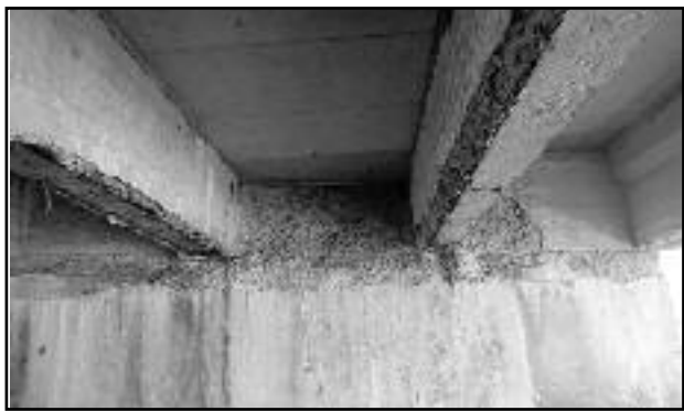
(above): Deterioration in deck under the Valley Road bridge.
